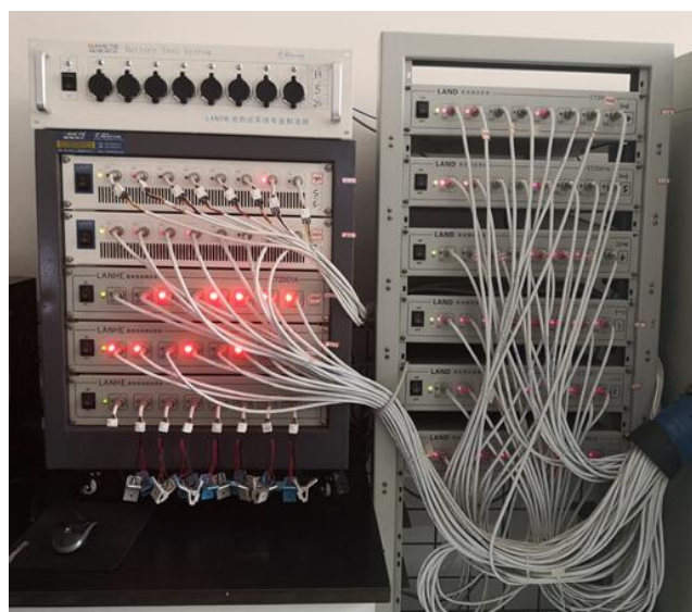
Fig.5 Battery test system.
